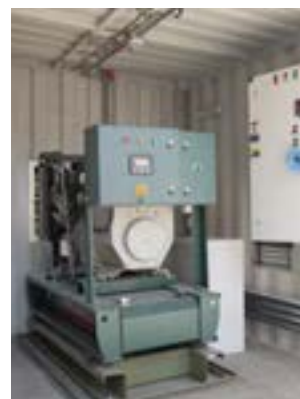
Generator Room / Genset Area
