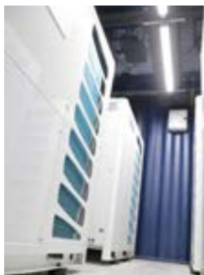
Cooling Room / Mechanical Room
