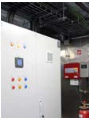
Power Room / Electrical Room (ER)
