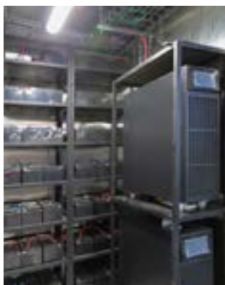
UPS Room & Battery Room
