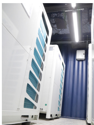
Cooling Room / Mechanical Room
