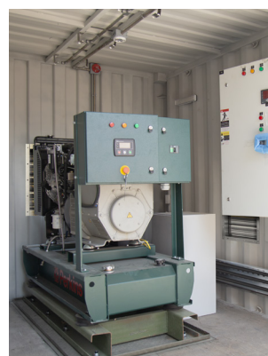
Generator Room / Genset Area
