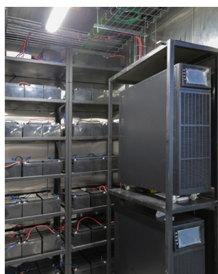
UPS Room & Battery Room
