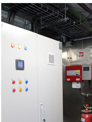
Power Room / Electrical Room (ER)
