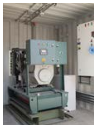
Generator Room / Genset Area
