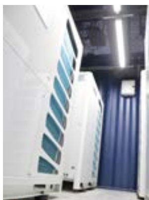
Cooling Room / Mechanical Room
