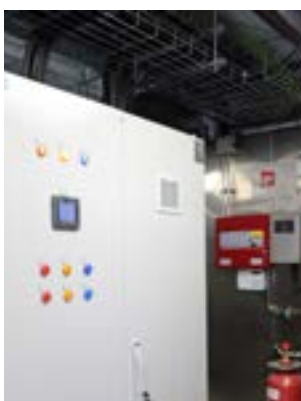
Power Room / Electrical Room (ER)
