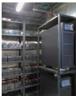
UPS Room & Battery Room
