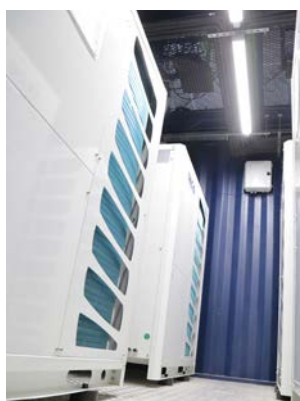
Cooling Room / Mechanical Room
