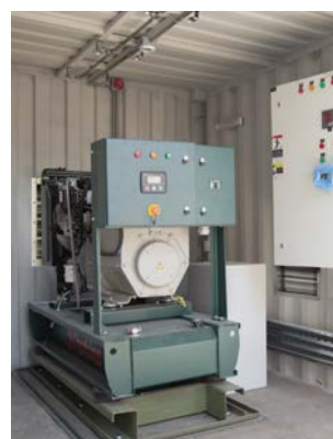
Generator Room / Genset Area
