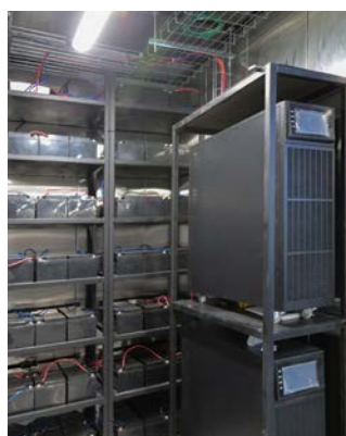
UPS Room & Battery Room
