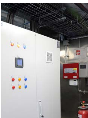
Power Room / Electrical Room (ER)
